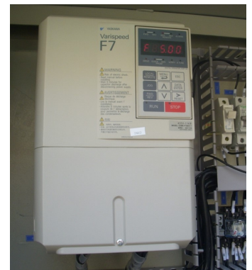
Inverters Yaskawa & Schneider Brand
