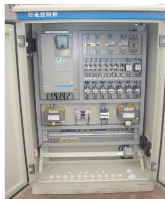
Trolley & Slewing Control Panel Box
